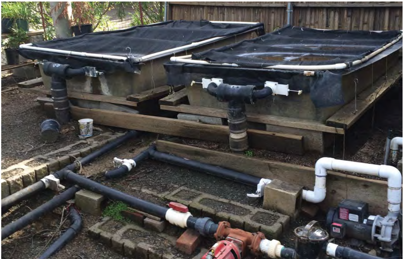
Existing filtration system at Koi Pond
